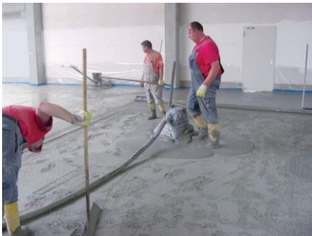
Application with pneumatic conveyor
